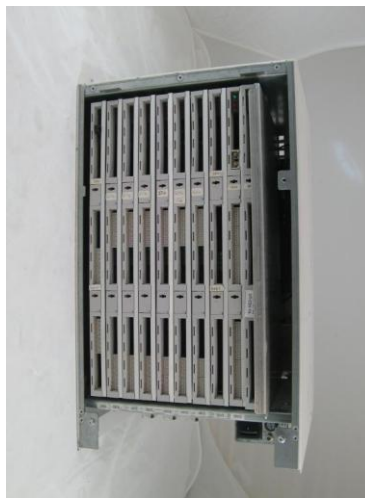
Figuur 8 Ericsson DECT Central Communication System
